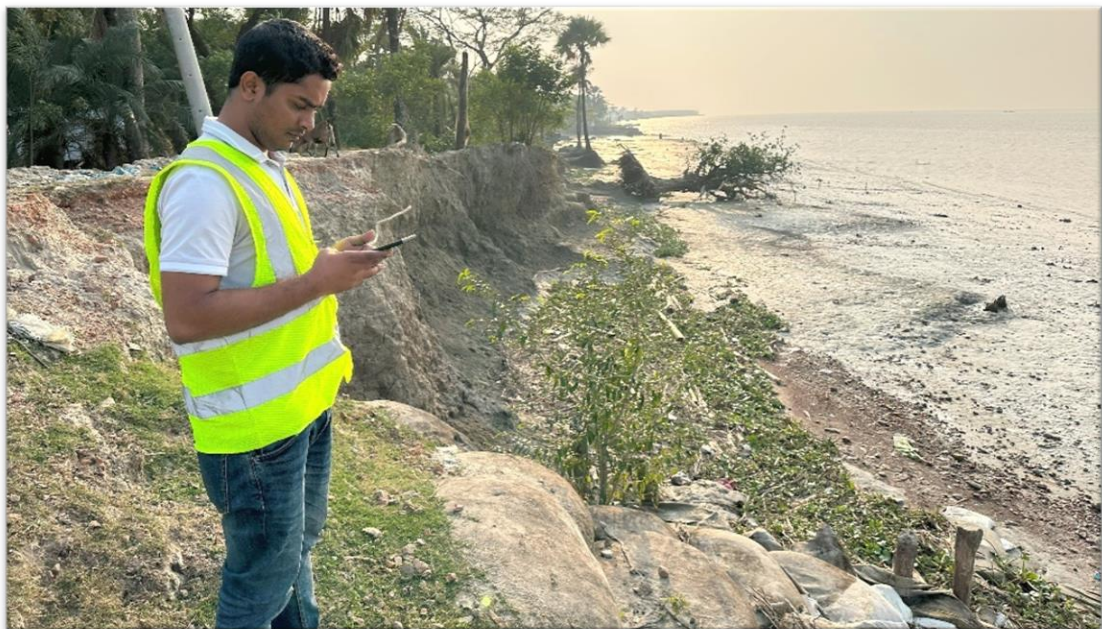
Figure 4: River erosion in Sonakata union
