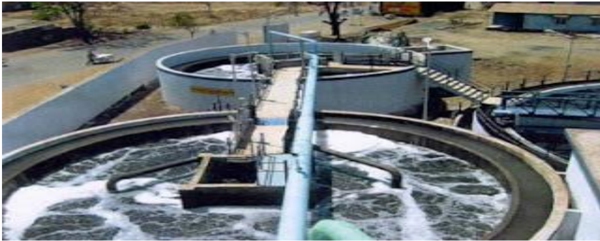
Figure 4: Effluent Treatment Plant (ETP)
