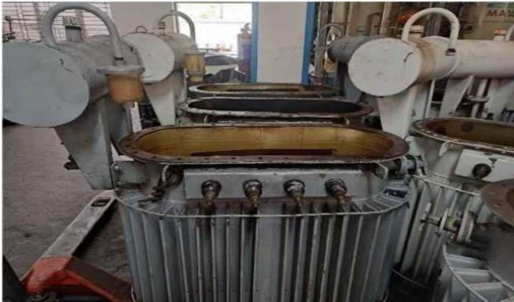
Figure 5.4: Radiator of Transformer
