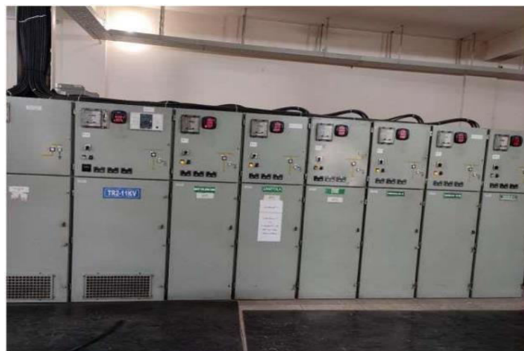
Figure 4.4: Control Room Substation
