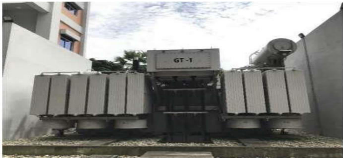
Figure 3.1: Transformer at Bashundhara Grid Substation
