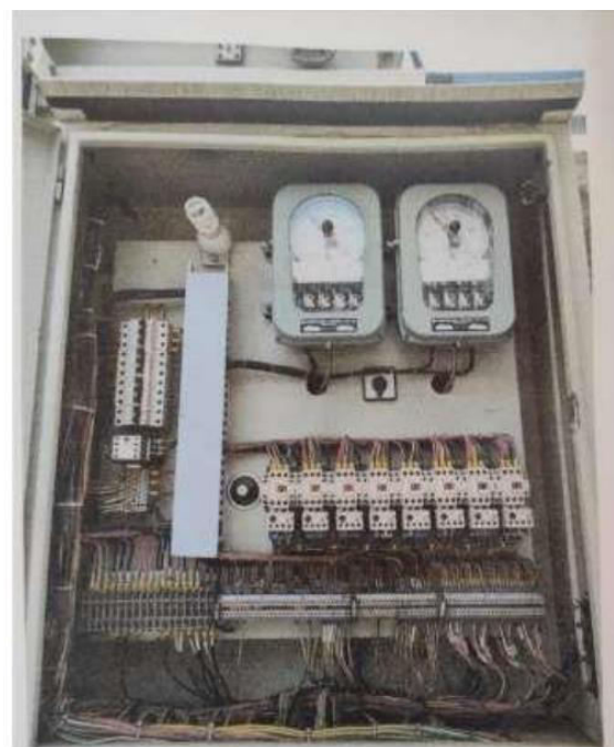
Figure 3.4: Winding temperature and Oil temperature indicator
