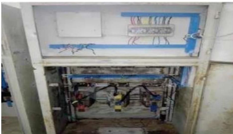
Figure 5.11: High Tension Current Transformer Meter
