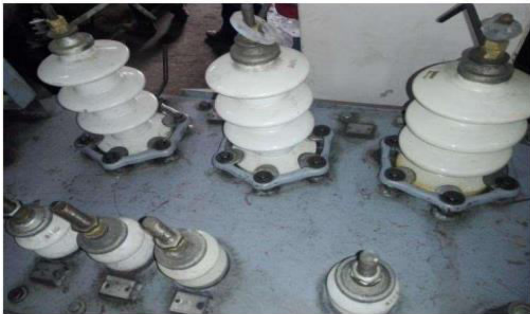
Figure 5.5: Bushing of Transformer
