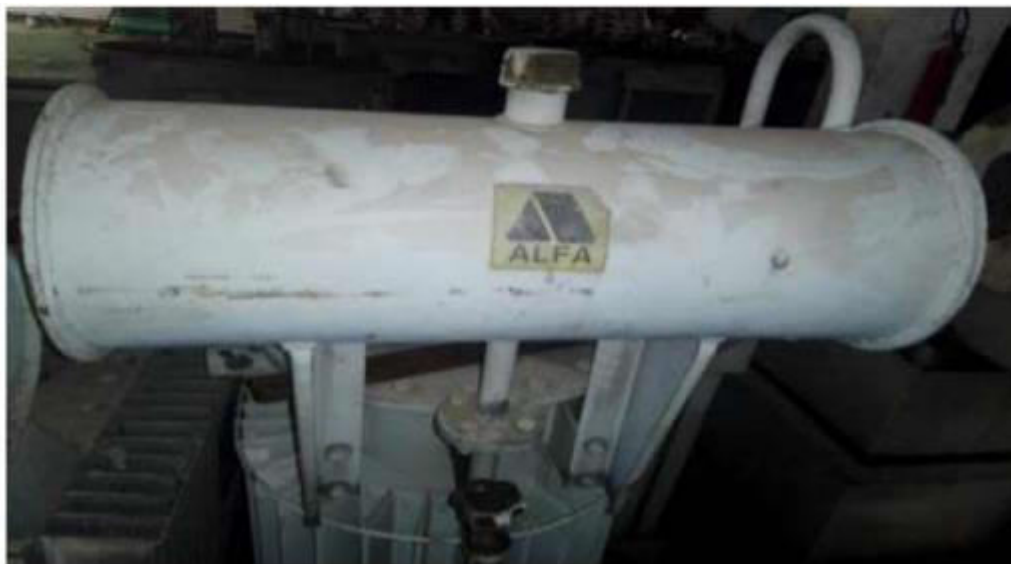
Figure 5.3: Conservative tank of Transformer
