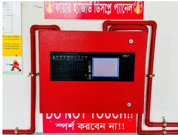
Figure 5.1: Running Fire Alarm Control Panel (FACP)
