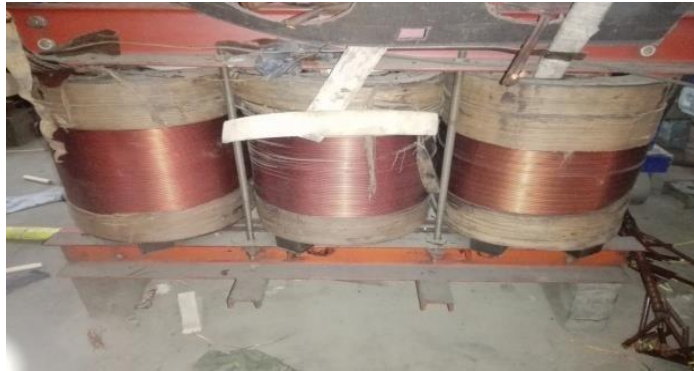
Figure 6.3: Coil of Transformer
