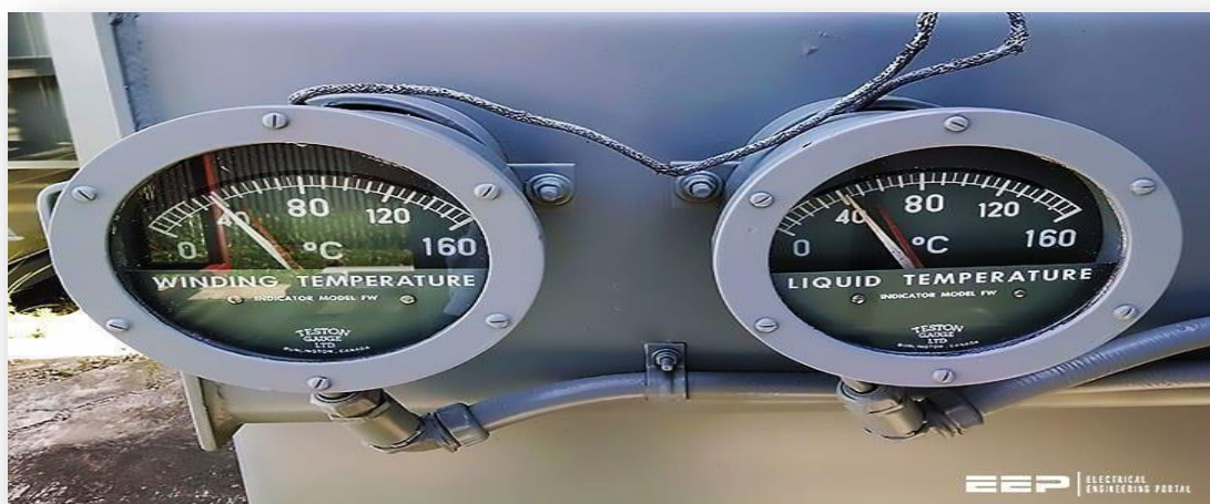
Figure 5.4: Winding temperature and oil temperature indicator
