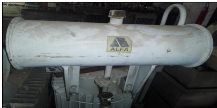
Figure 6.4: Conservative tank of Transformer
