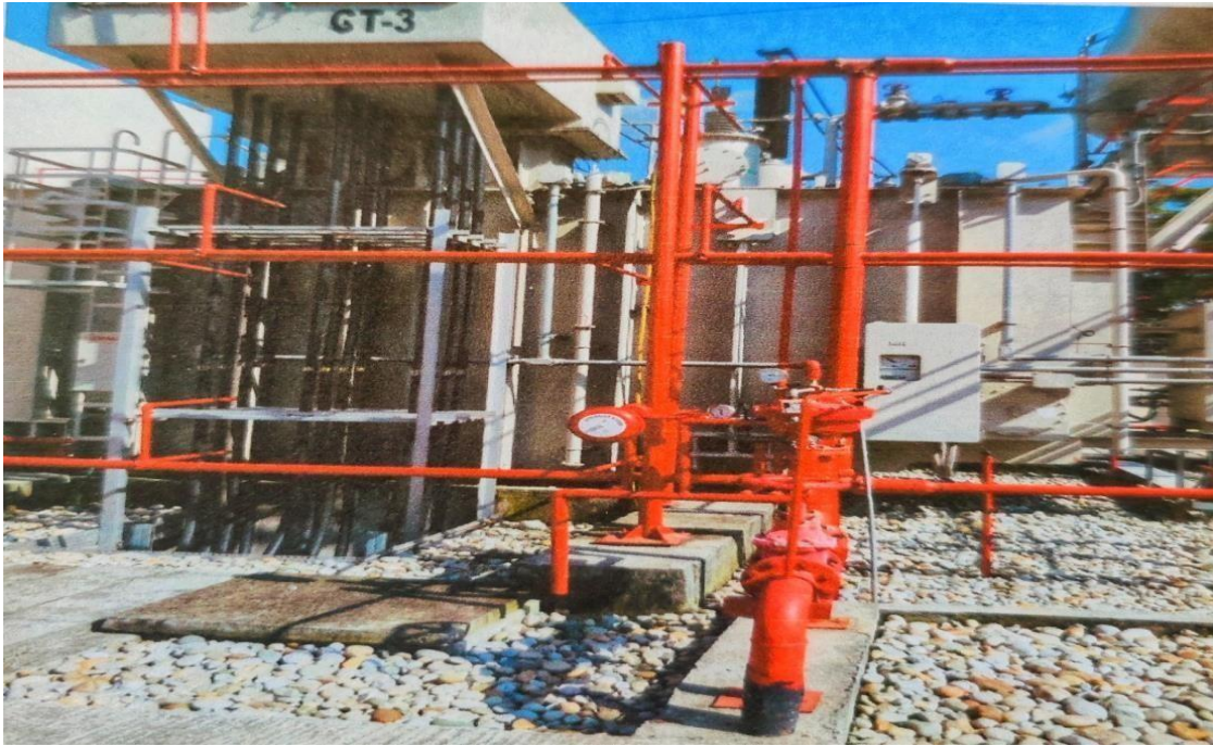
Figure 4.6 Lake City 132/33 KV Grid Substation
