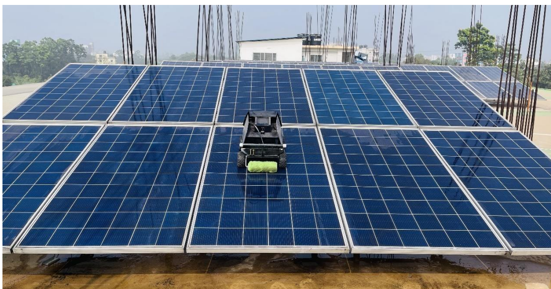
Fig. 4.3: Solar Panel Cleaning Process
