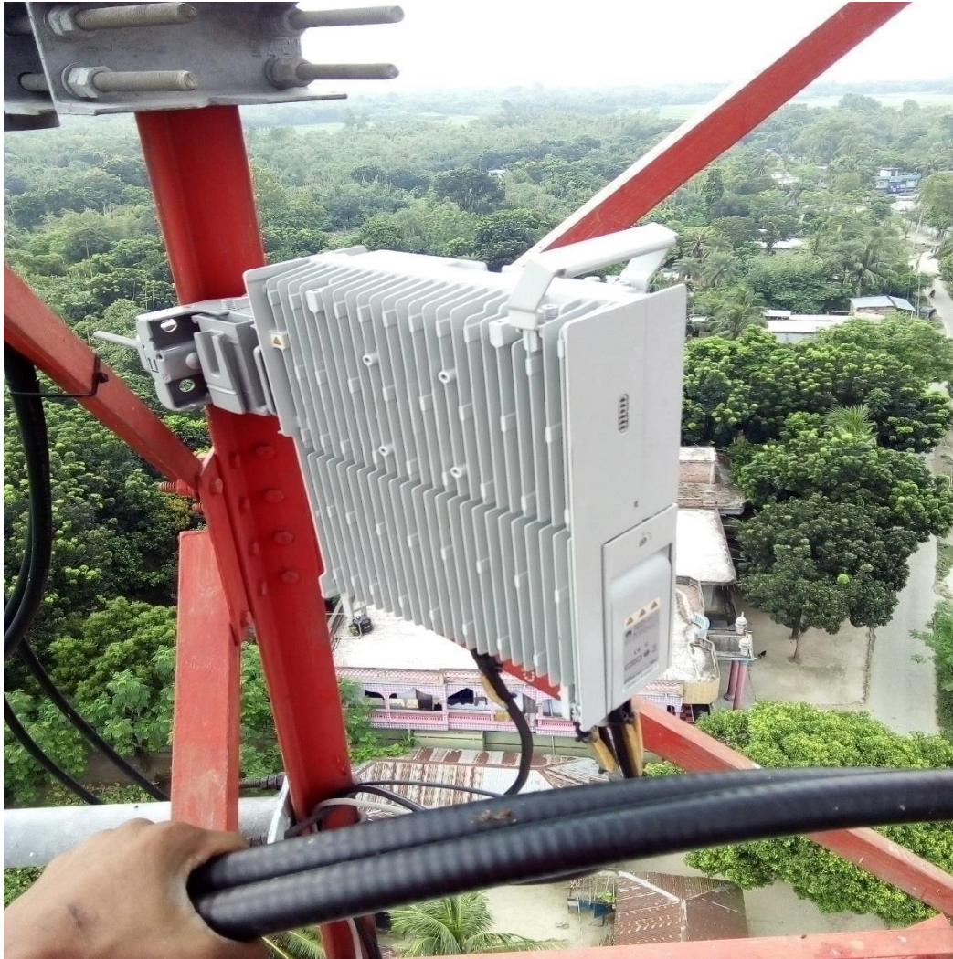
Fig5.12: RRU on BTS
