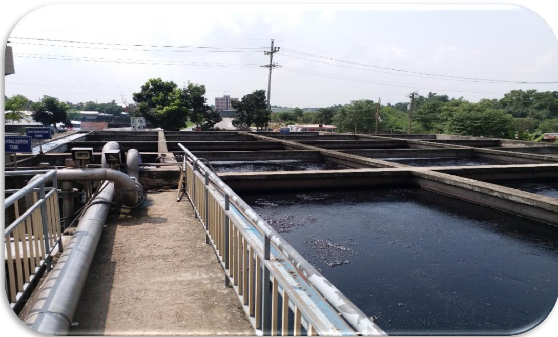
Effluent Treatment Plant
