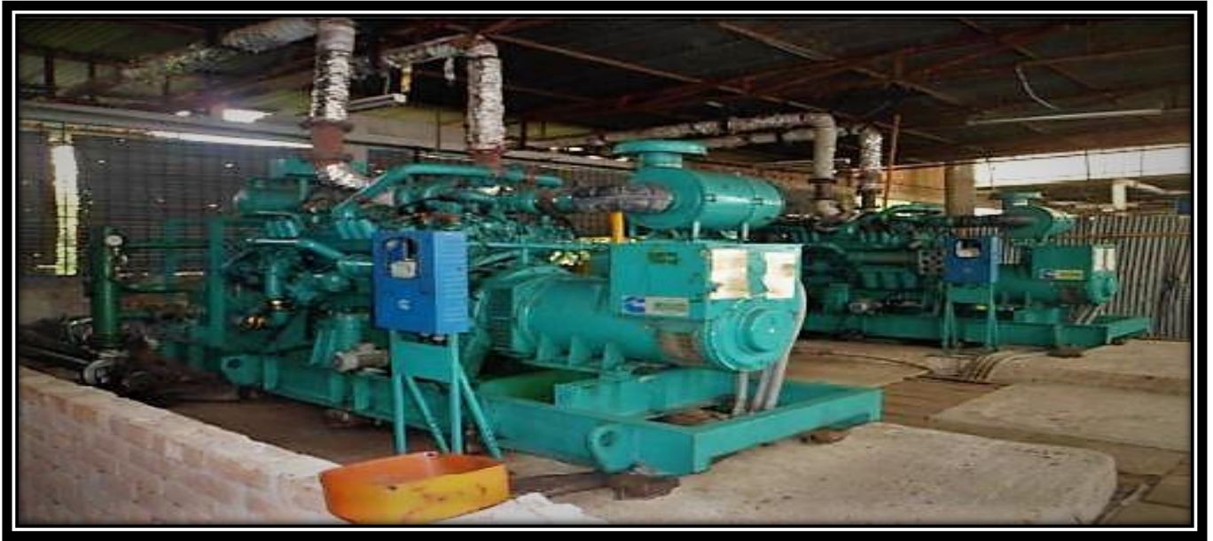
Figure: Gas Generator
