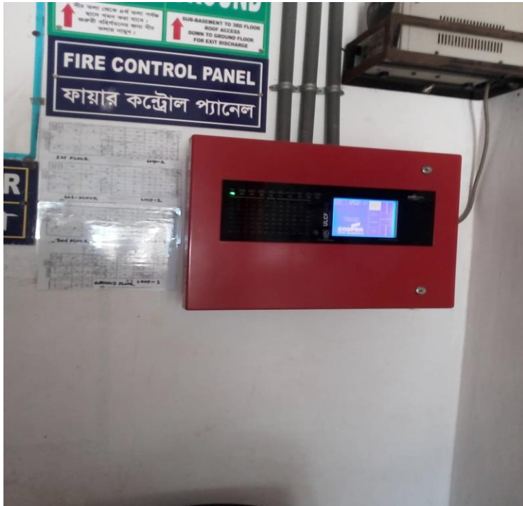
Picture 3.6.3.2. Fire control panel
