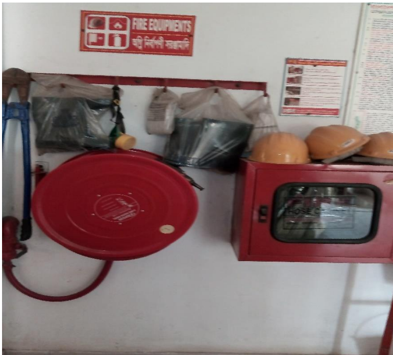
Picture 3.6.3.1. Fire equipment
