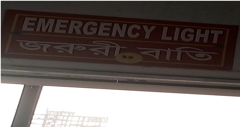
Picture 3.6.6.2. Emergency light
