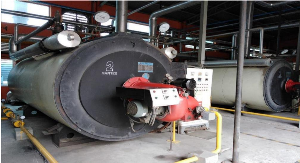
Figure 3.11. 5 Hot Oil Boiler
