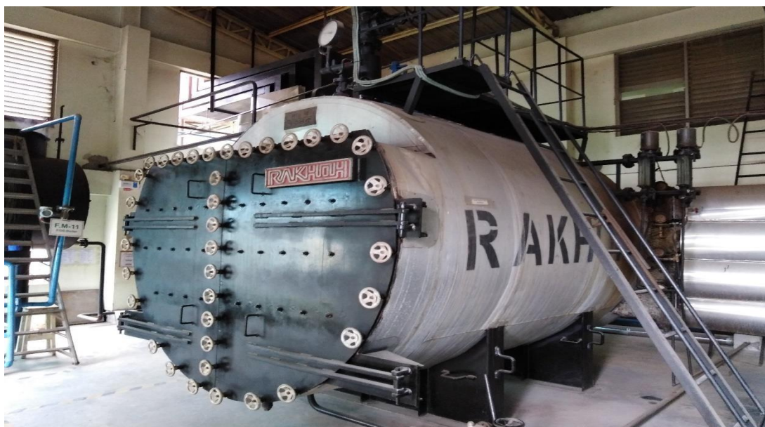
Figure 3.11. 6 Exhaust Gas Boiler
