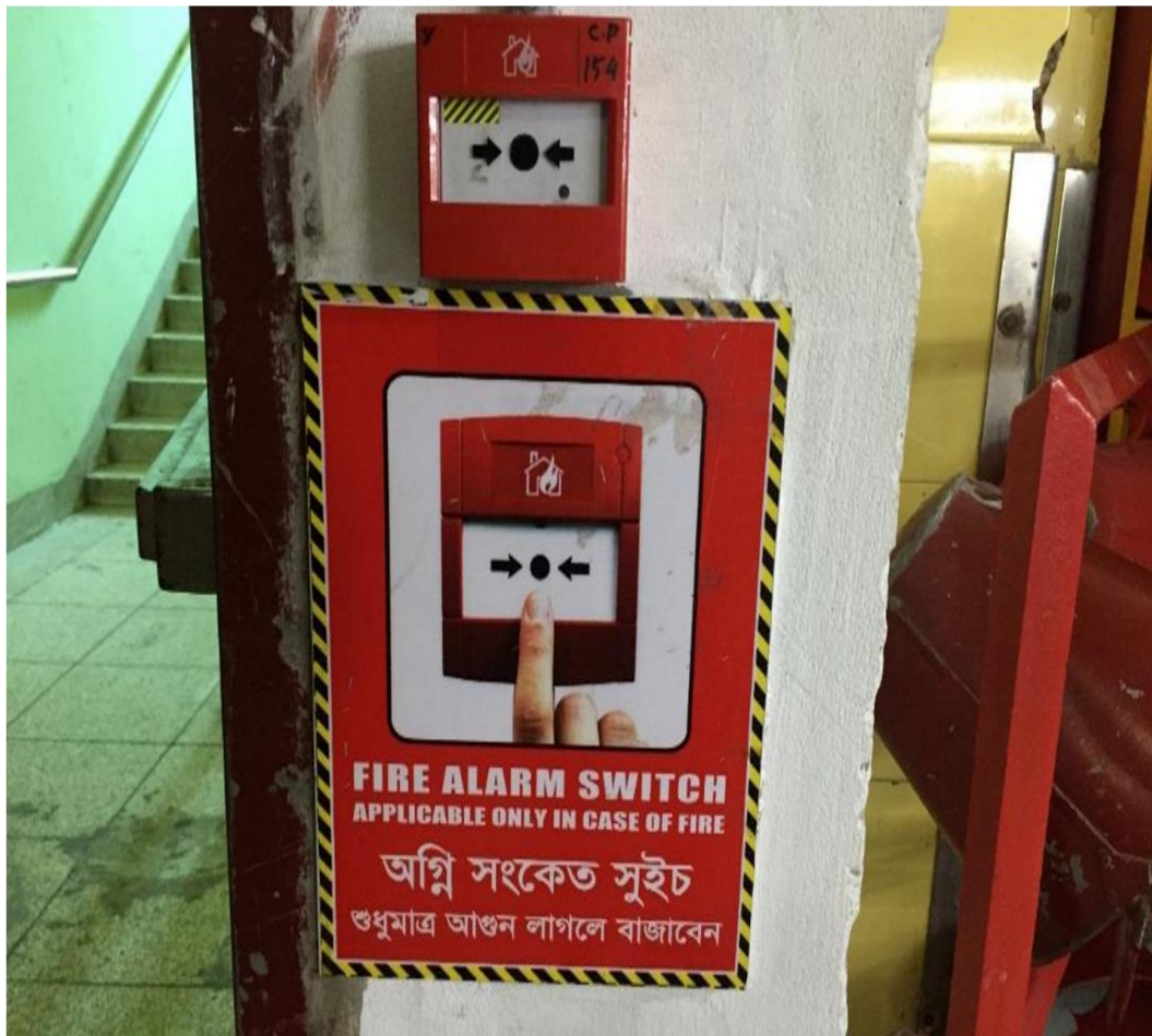
Figure 3.13. 9 Fire Alarm Switch
