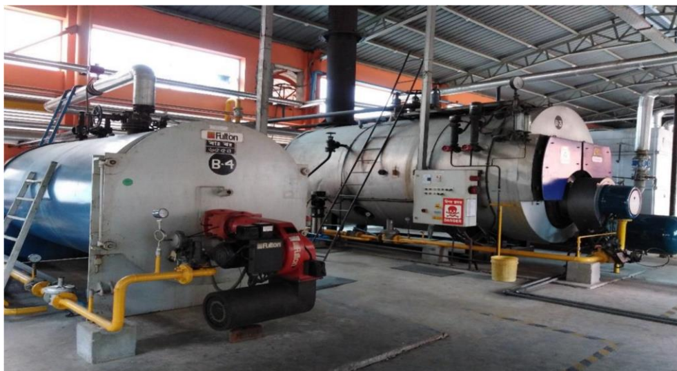
Figure 3.11. 4 Natural Gas Boiler
