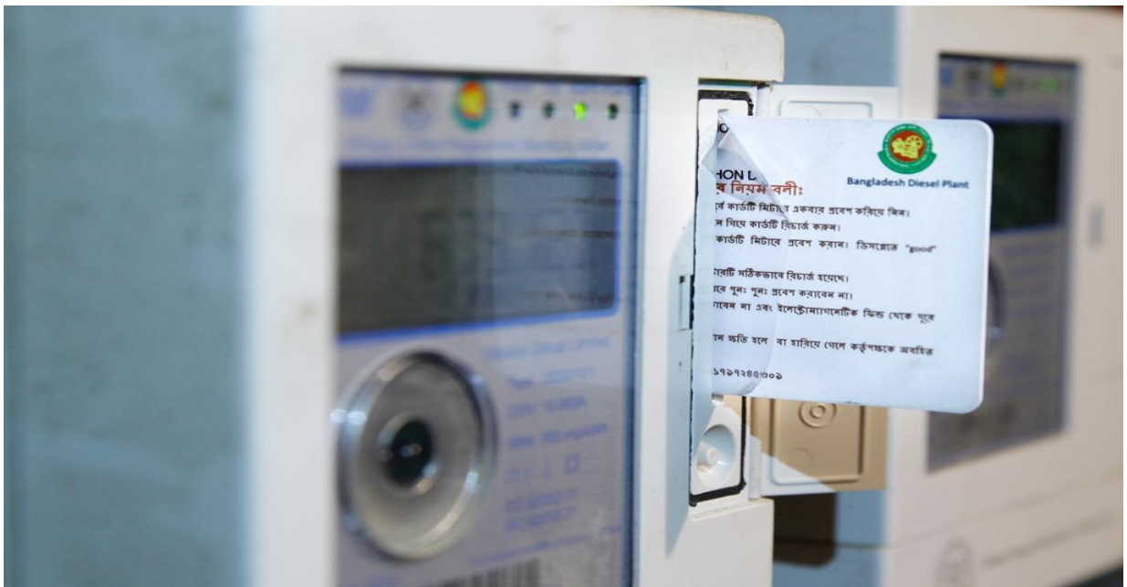
Fig 6.6: Prepaid Energy Meter
