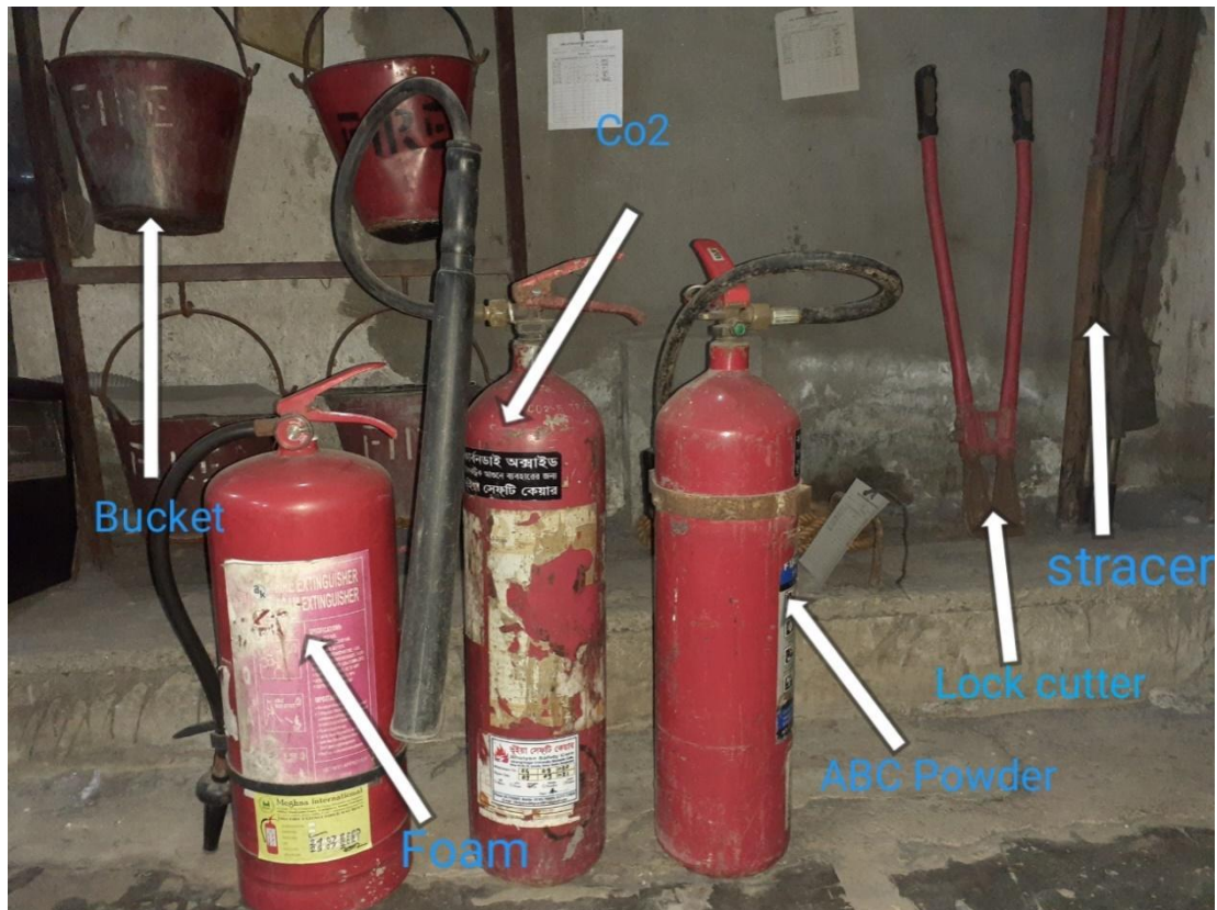
Fig: 11.2 Fire Extinguishers.
