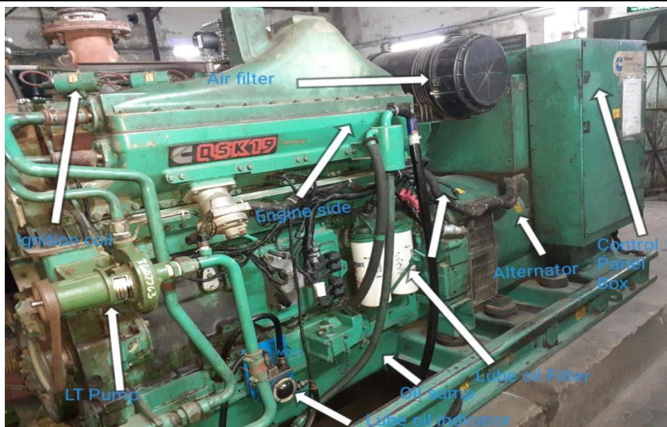
Fig: 4.1 Gas Generators left side.
