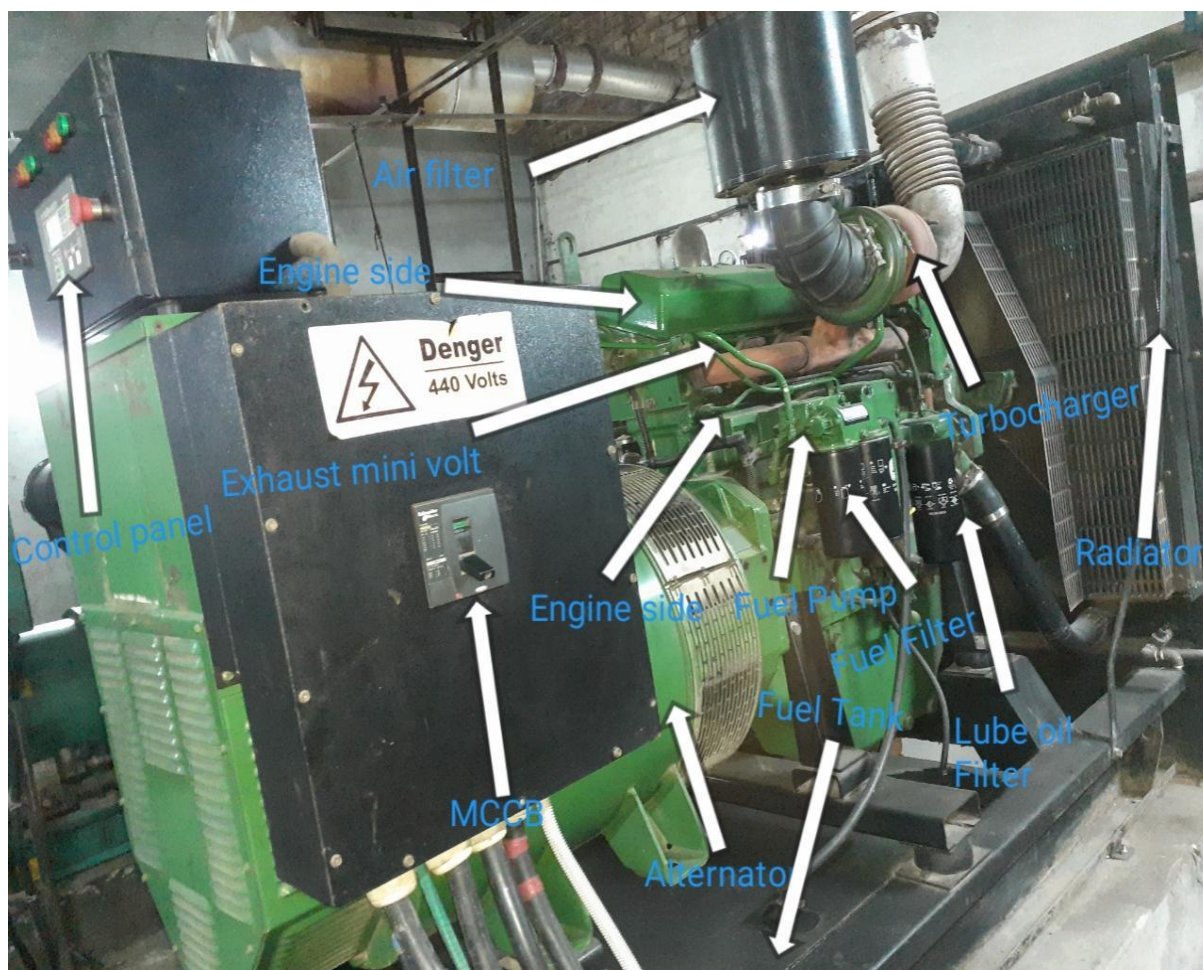
Fig: 3.5 Diesel Generators.
