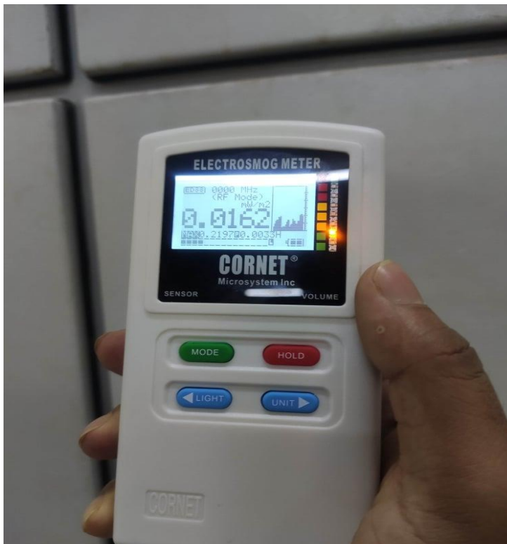
(We using Directional ELECTROSMOG meter at Power Substation)
