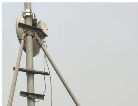
Figure 9.2: BTS Antennas on Cell Tower
