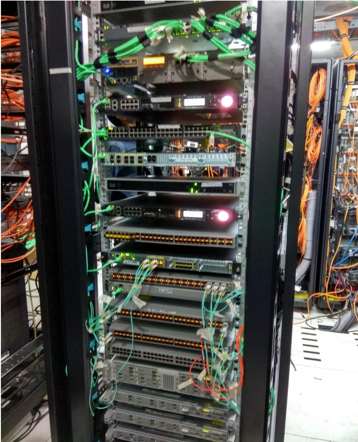
Figure 5.8 : Data Center ABL
