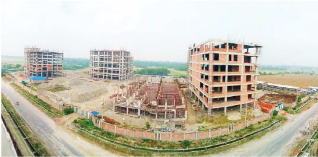
Present Panorama view of API Project
