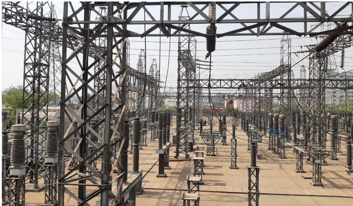
Figure 3.12: Kamrangirchar (132/33/11) KV Grid
