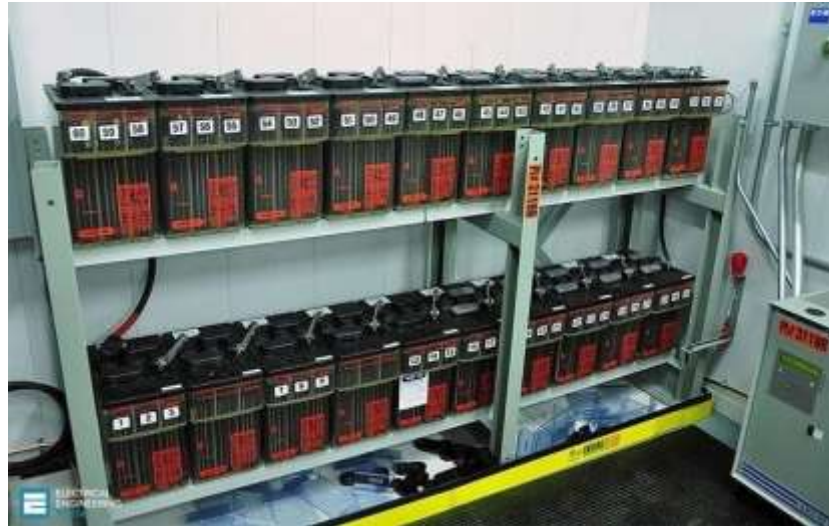
Figure 4 Battery and Battery Charger.
