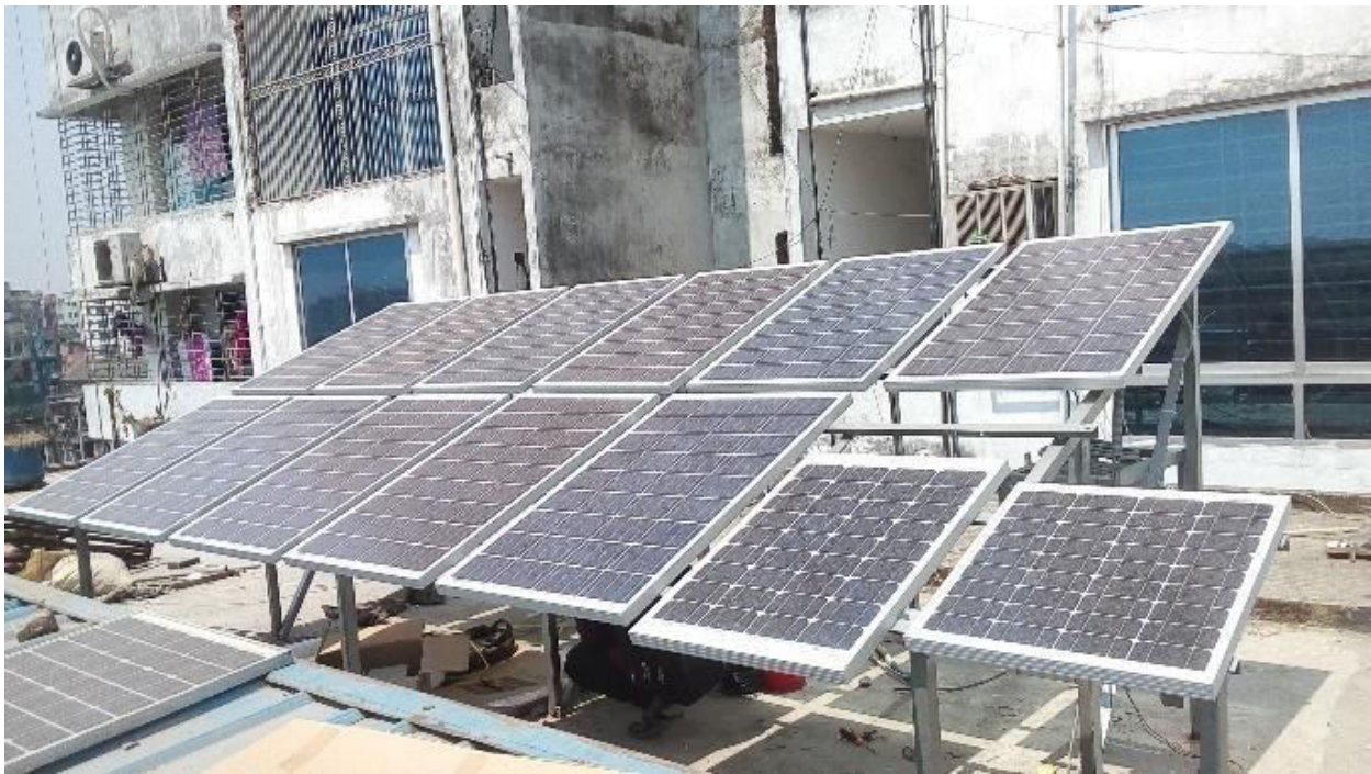
Fig. 4.1: Off & On Grid Solar System on Rooftop of Daffodil International University
