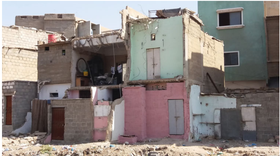
Fig. 12 Half demolished structure being used as living space
