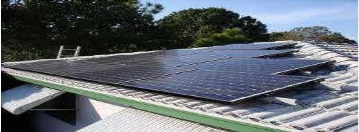
Figure 2.19. Fin mounting on roof
