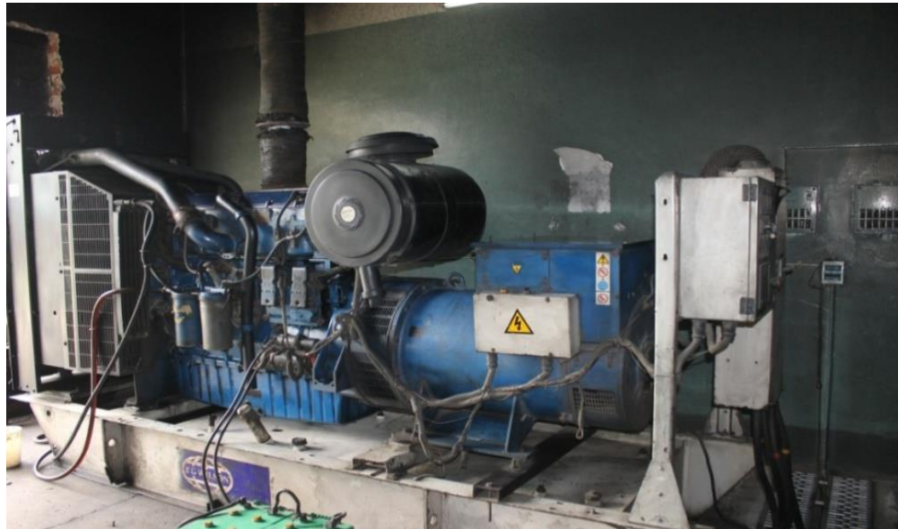
Fig 2.1 Diesel Generator (Perkins)
