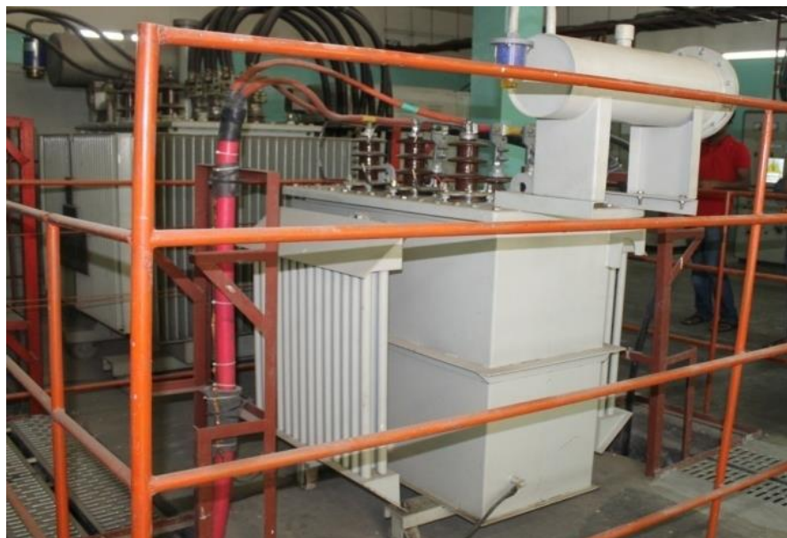
Figure 3.1 :11000/415V, 3-Phase distribution transformer
