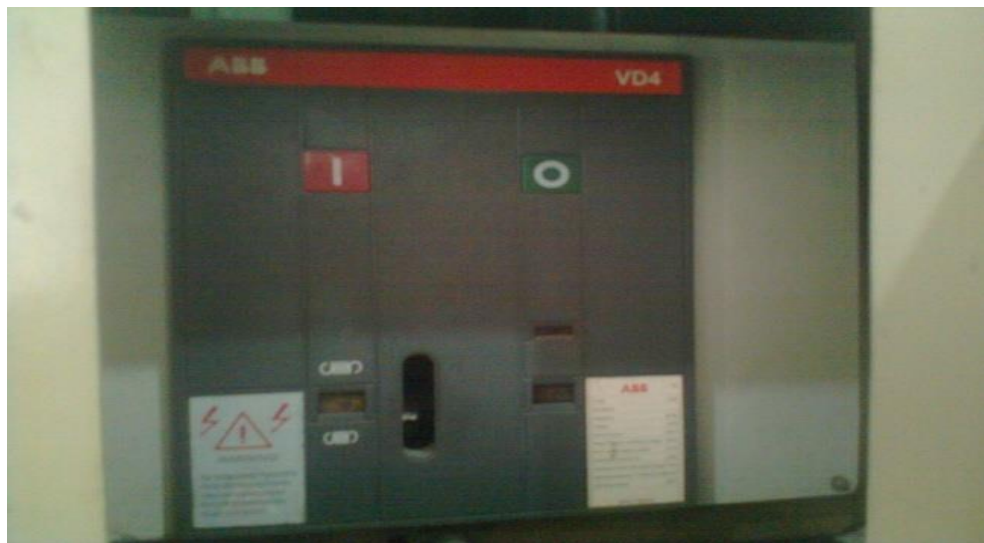
Figure 4.1 Vacuum circuit breaker (VCB)
