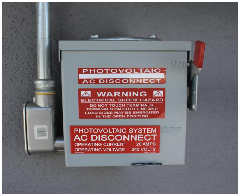
Figure 2.18: AC Disconnect (Utility Accessible)
