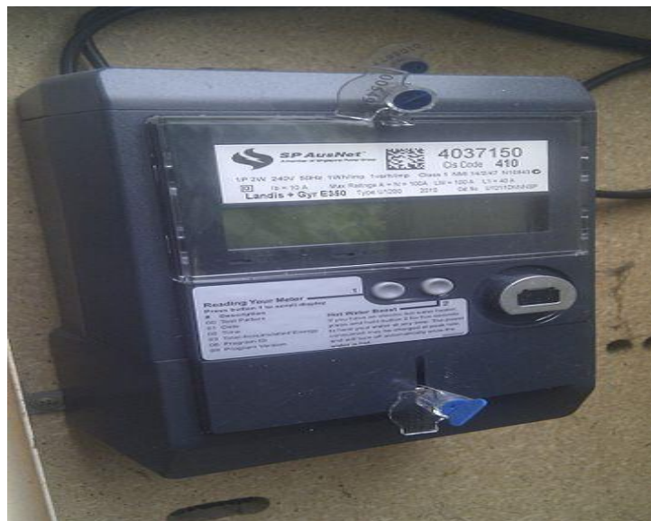
Figure 2.19: Net meter of solar PV
