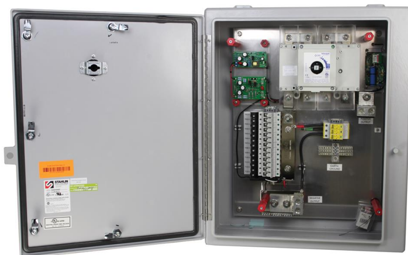
Figure 2.15: Combiner box of solar PV
