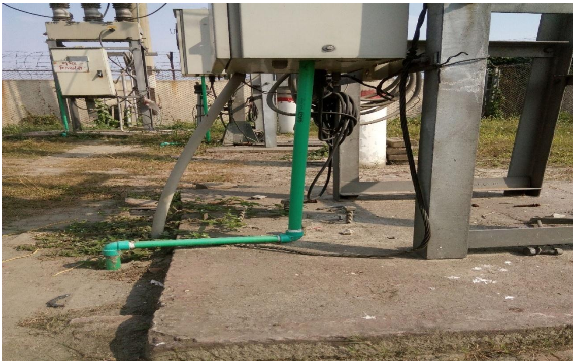
Fig. 3.5: Underground cable of NPBS-1 substation.
