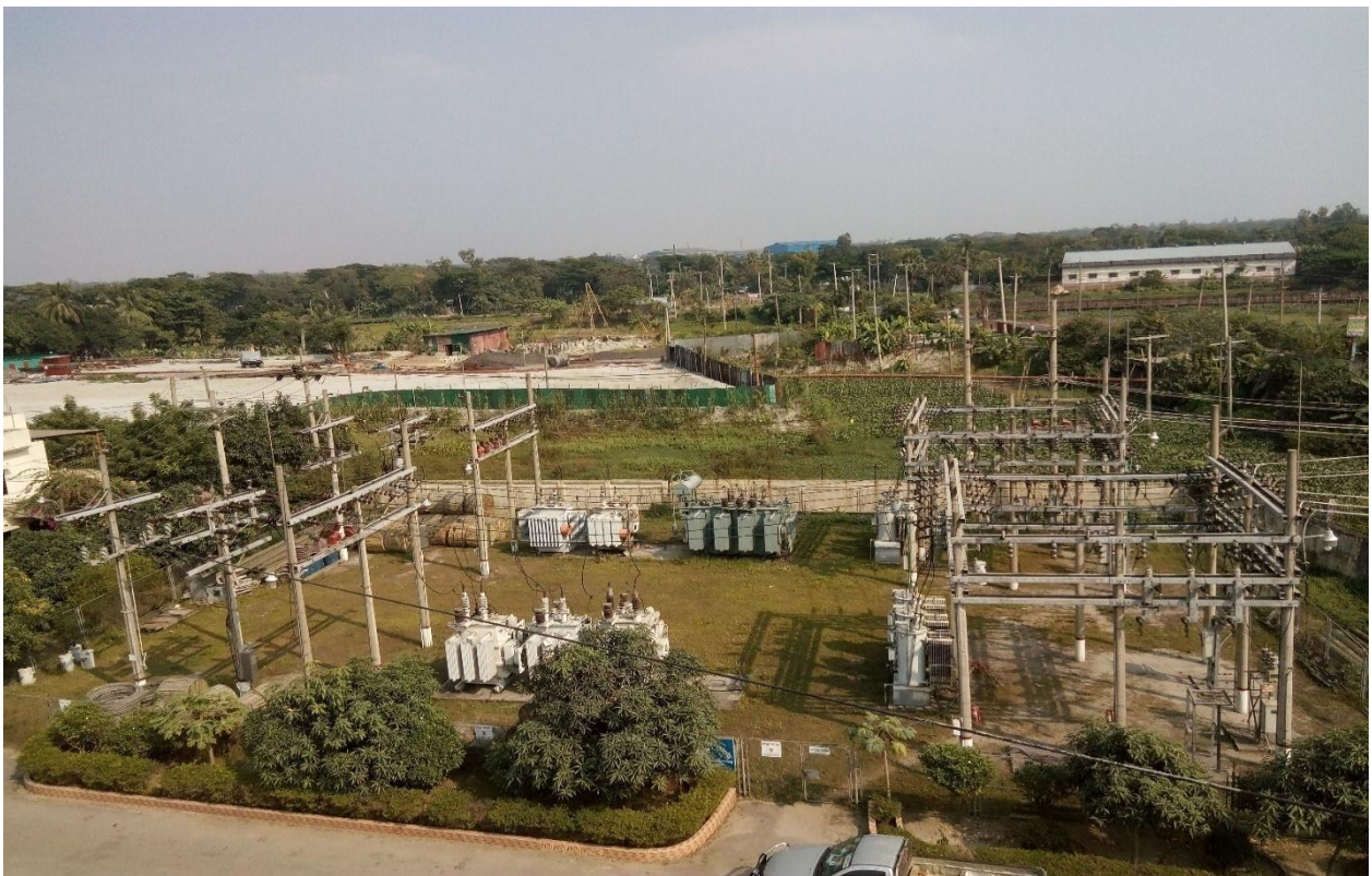
Figure 3.1: The substation of NPBS-1
