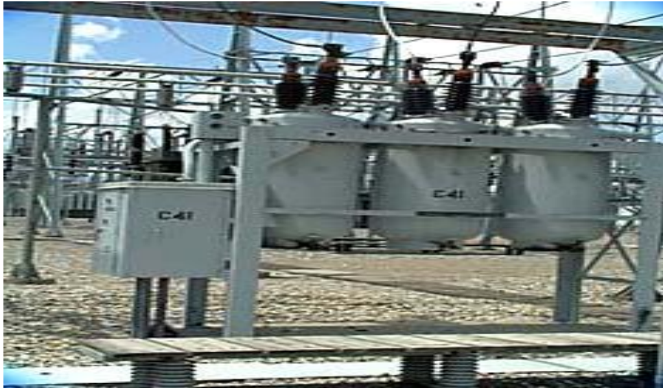
Fig. 5.2: Oil Circuit Breaker
