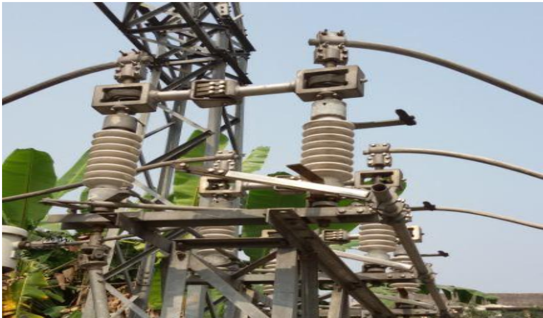
Fig. 3.4: Insulators used in NPBS-1 substation
