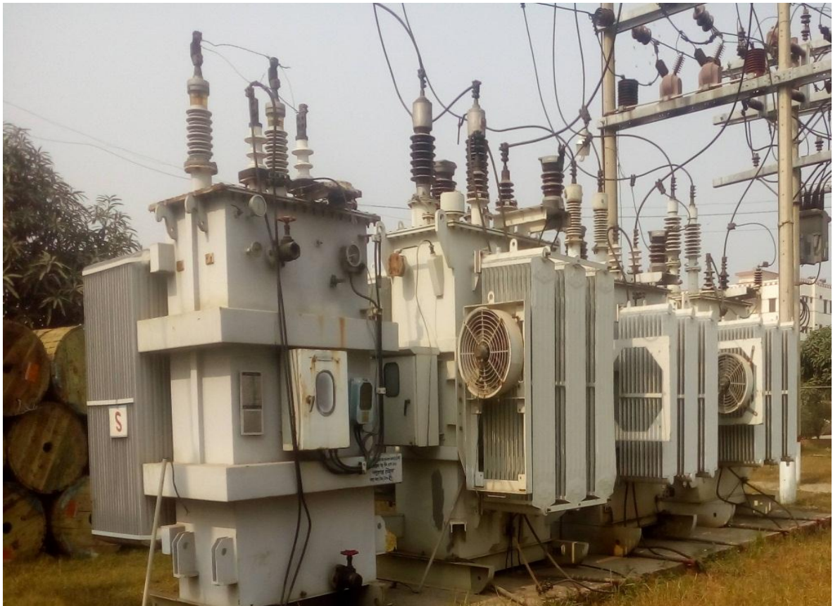
Fig. 3.2: Power transformer of Narayanganaj PBS-1
