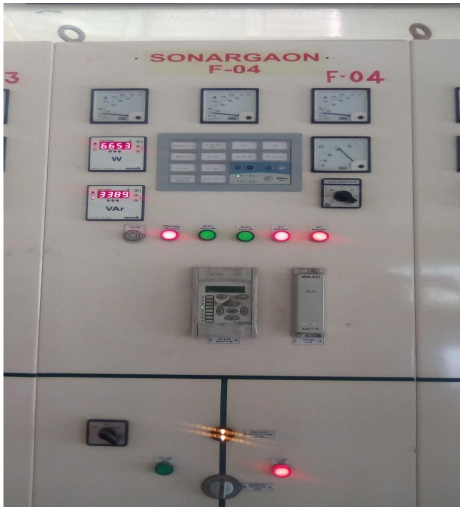
Fig. 5.1: Switchgear of NPBS-1 (Sonargaon)
