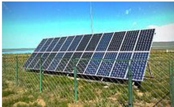
Figure 3.1 A solar array composed of a solar panel with 24 solar modules in rural area.
