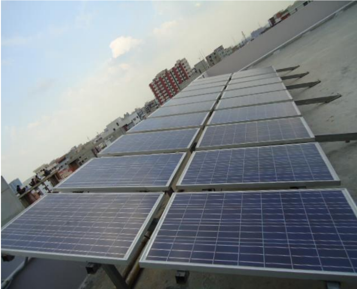
Fig: 2.16 solar rooftop system
