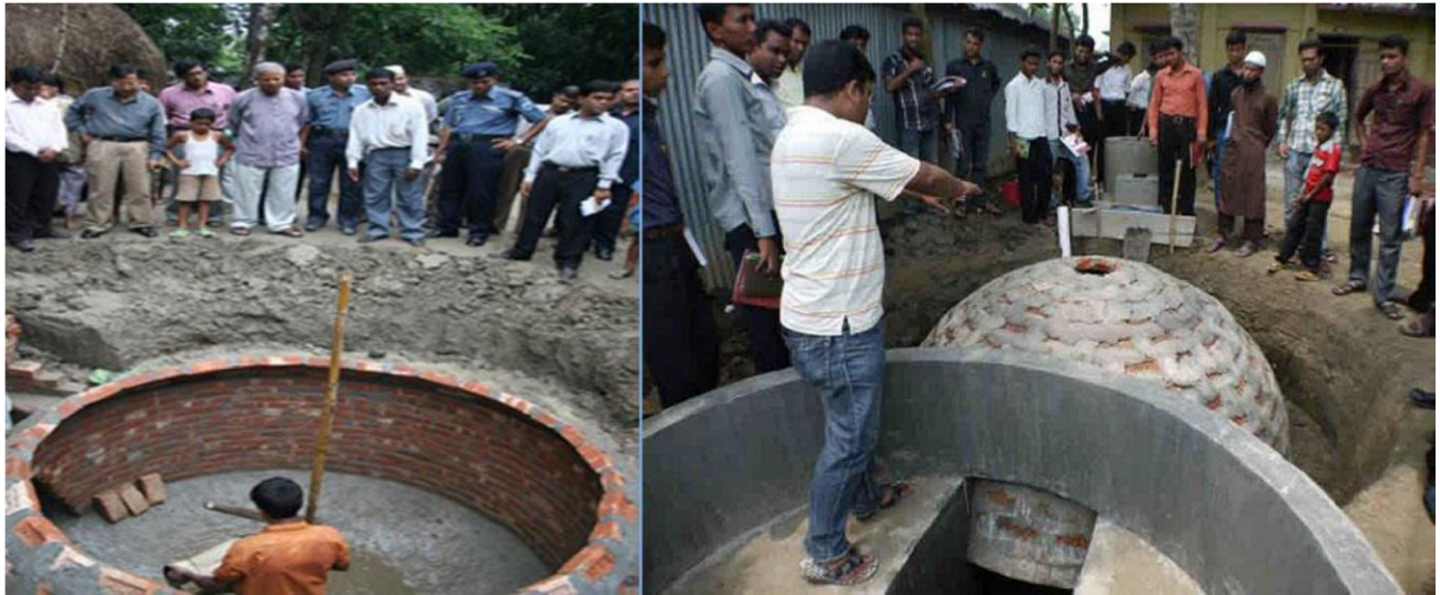
Fig-2.3: Biomass gas plant
