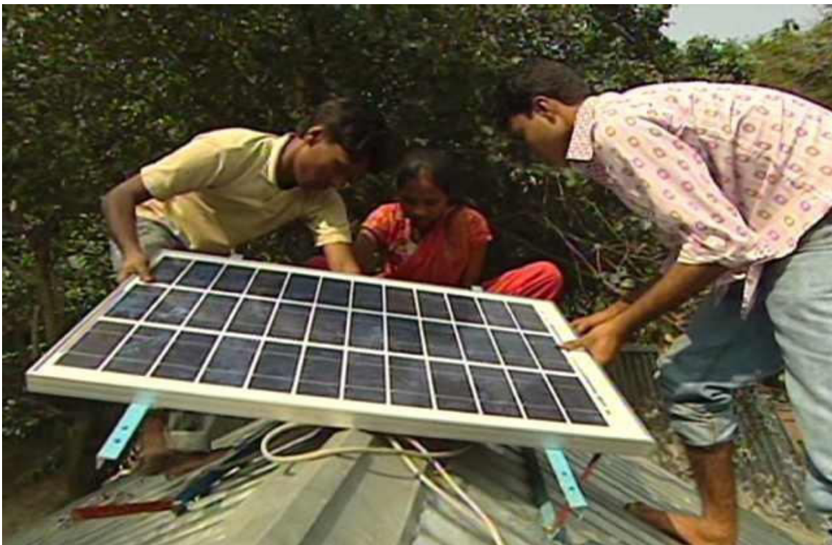
Fig-2.6: Rooftop Solar home system
