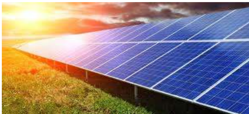
Figure 2.2: Solar energy collected by solar Panel
