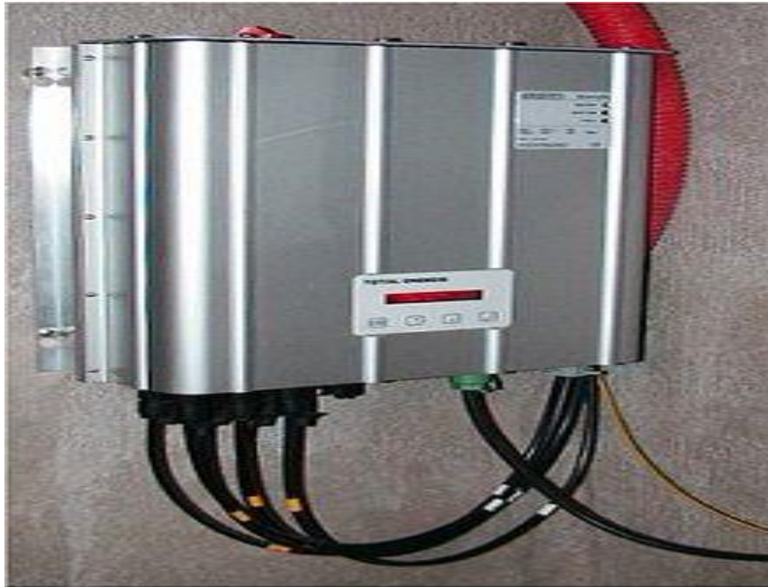
Figure 2.10: Inverter for grid connected PV
