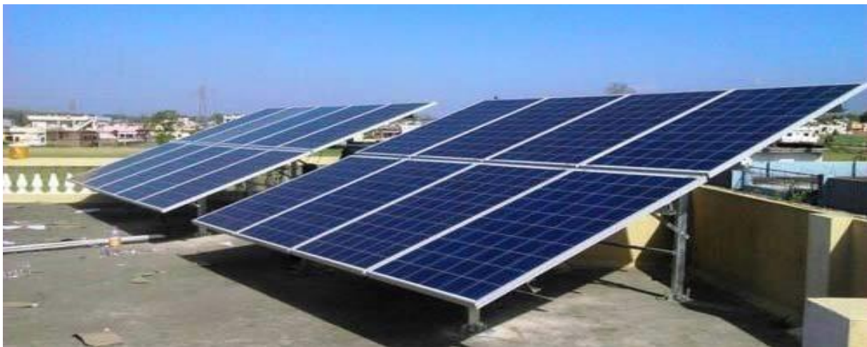
Figure 1.1: solar rooftop system at Narangonj
