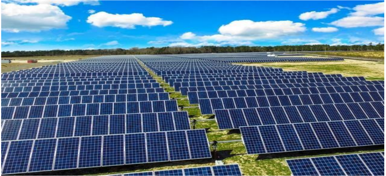
Figure: 2.1 Solar farm in Cox's bazar
