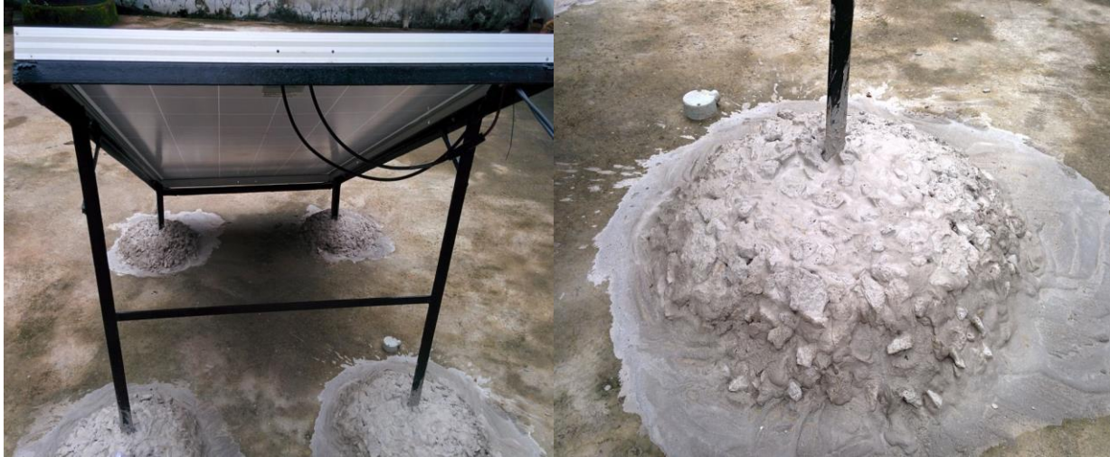
Fig 2.11: Solar panel mounting
