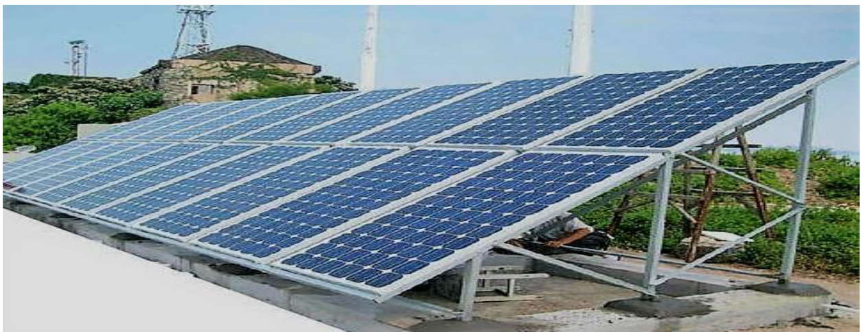
Figure 2.13: Solar PV modules
