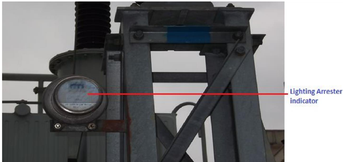
Figure 4.9: Lighting arrester indicator at Mogbazar grid-substation.
