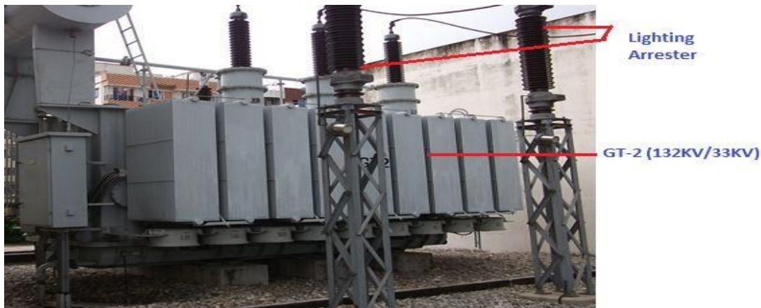
Figure 4.8: Lighting Arrester and GT-2 at mogbazar grid-substation.
