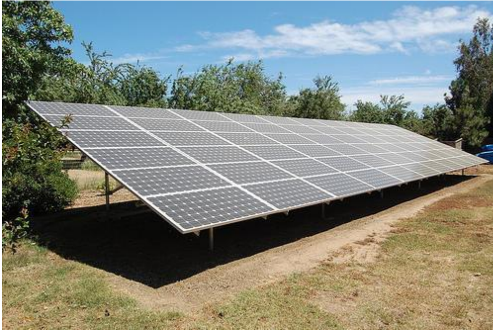
Fig 2.5 off grid solar panel
