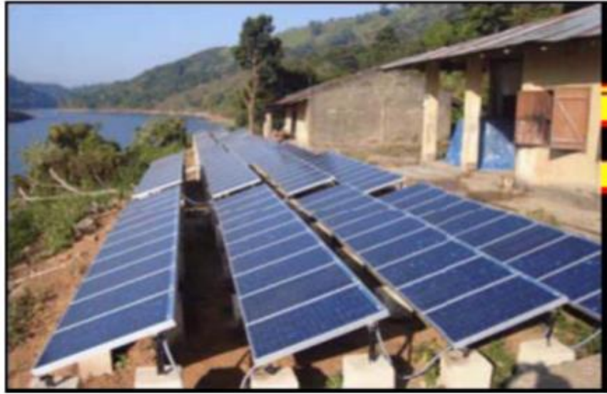
Figure 2.7: 10kw solar electrification systems at Barkal,Rangamati
