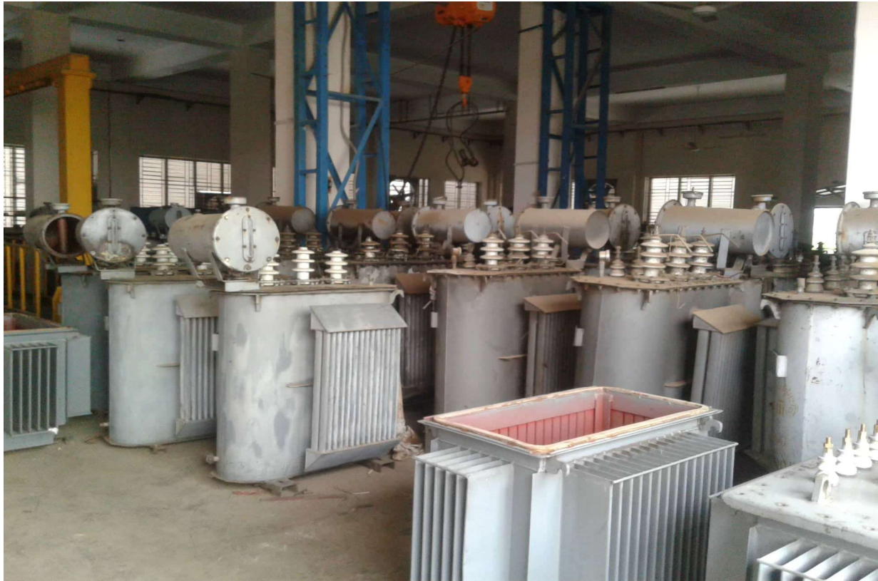
Figure: 2.4: Transformer Testing & Repairing Lab (DESCO).
