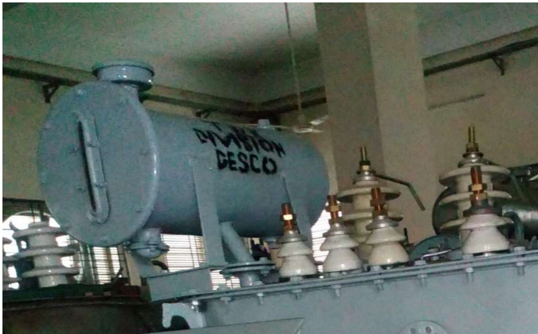
Figure: 3.16: Conservator tank.
