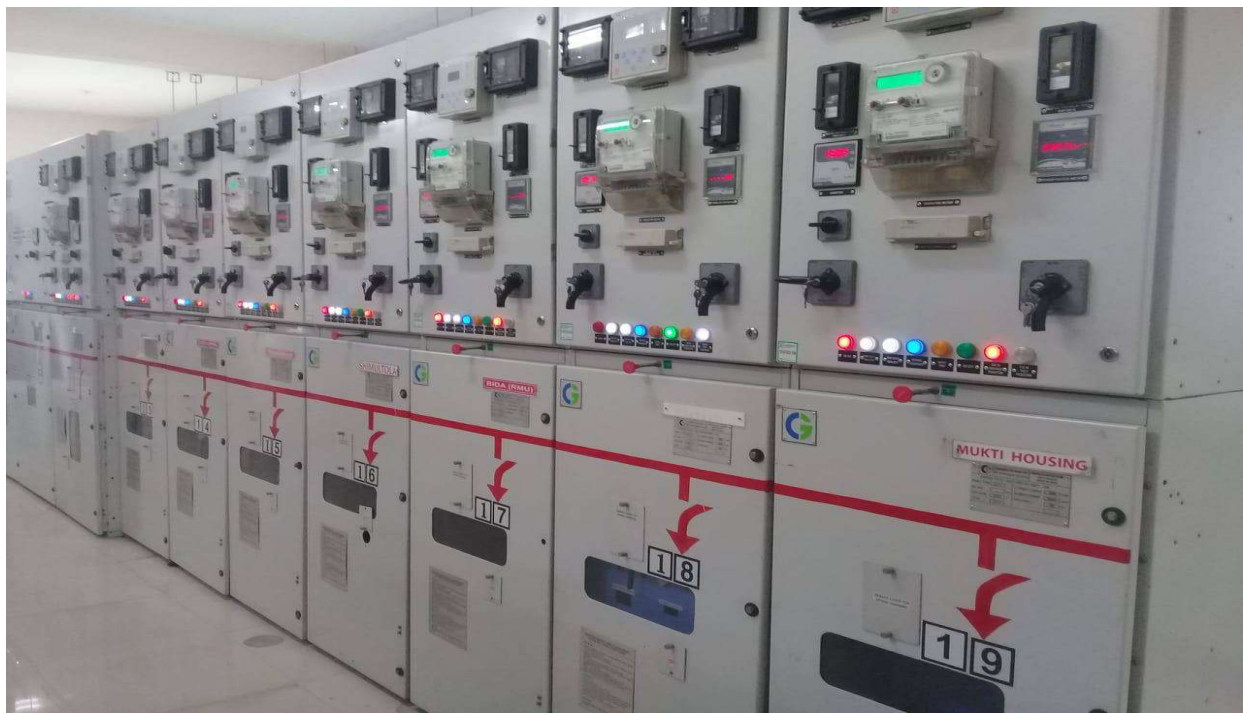
Figure: 3.3: Control Panel
