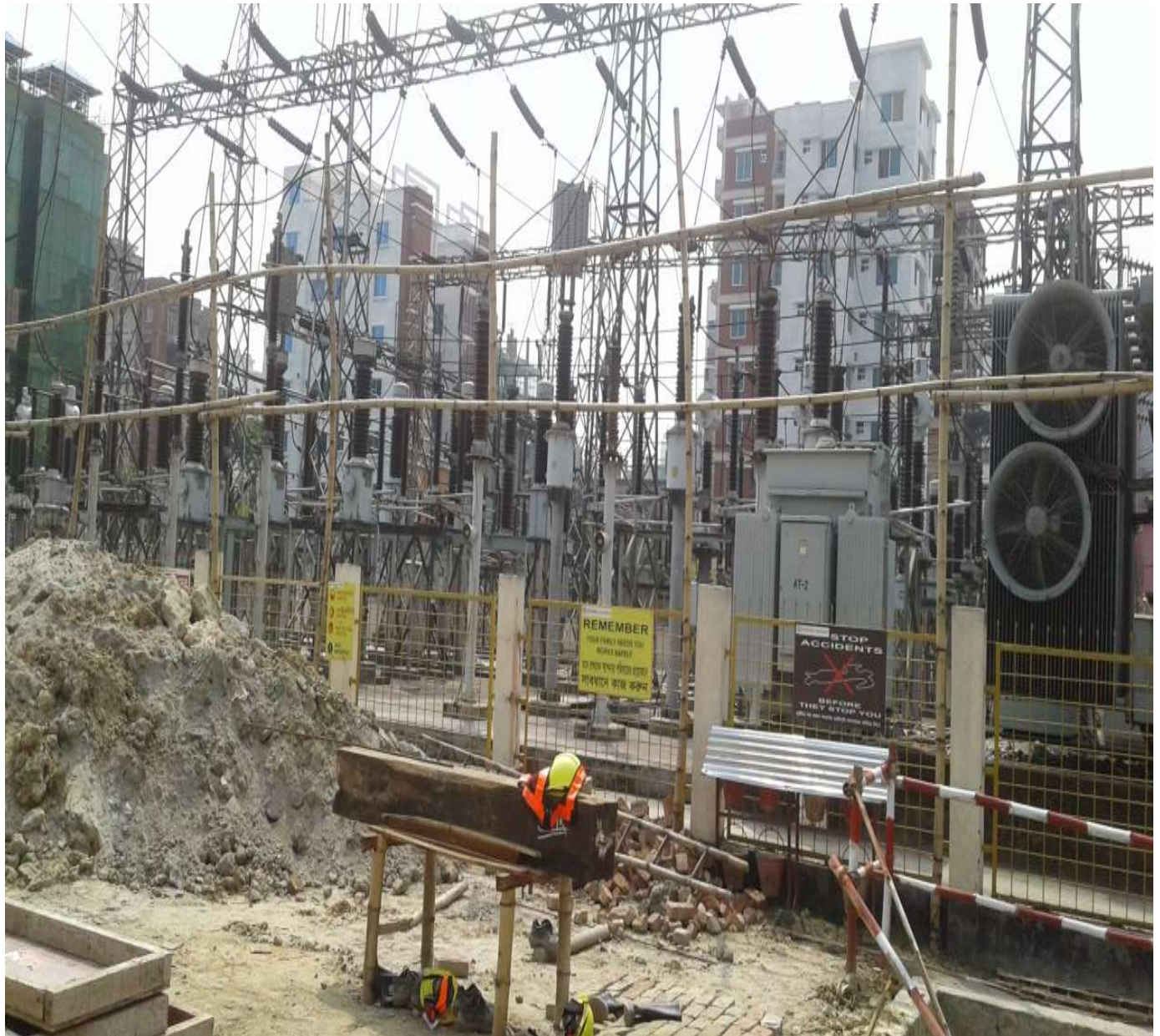
Figure: 2.2: AIS substation ( Bashundhara 132/33KV )
