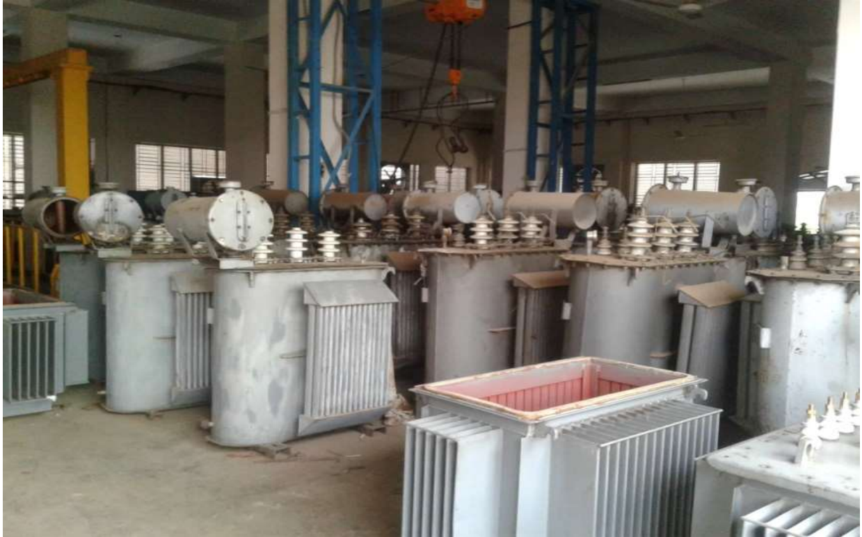
Figure: 3.20: Transformer Testing & Repairing Lab (DESCO)
