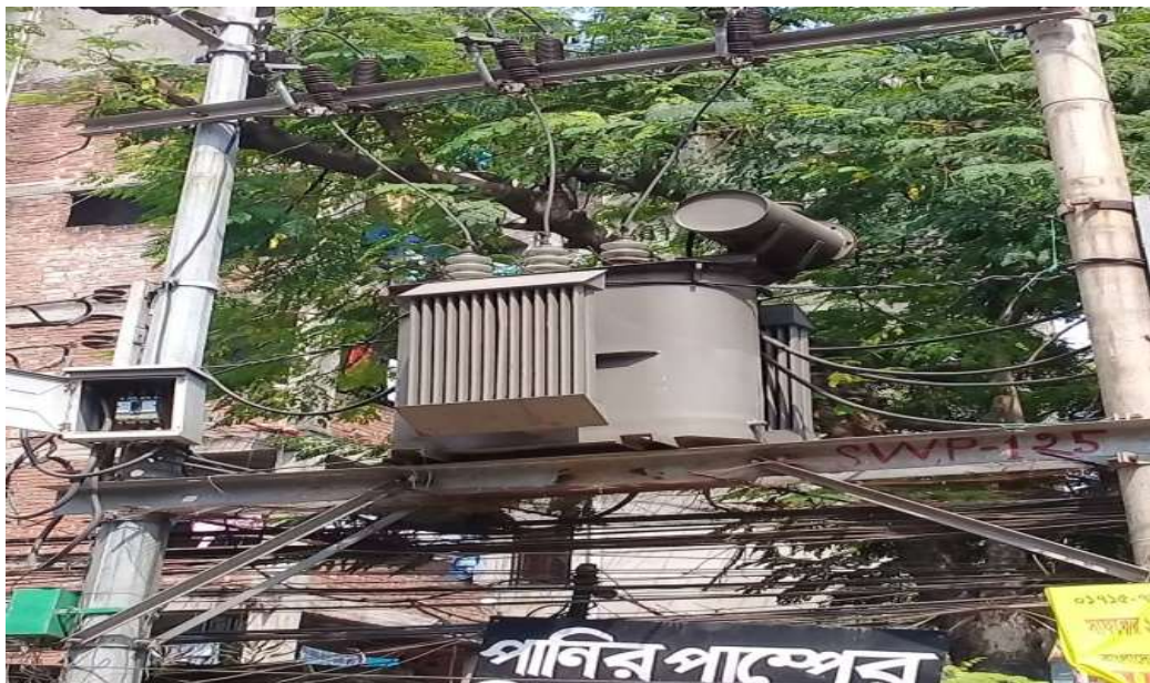
Figure: 3.11: Transformer Maintenance
