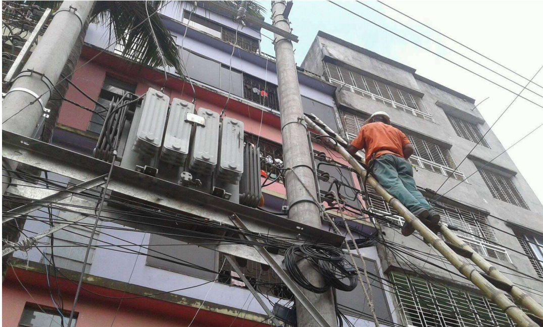
Figure: 3.12: Overhead Line Maintenance
