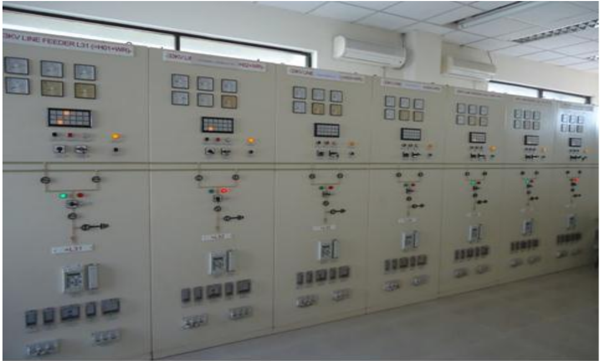
Figure- 3.9 Control room & Panel Boa
