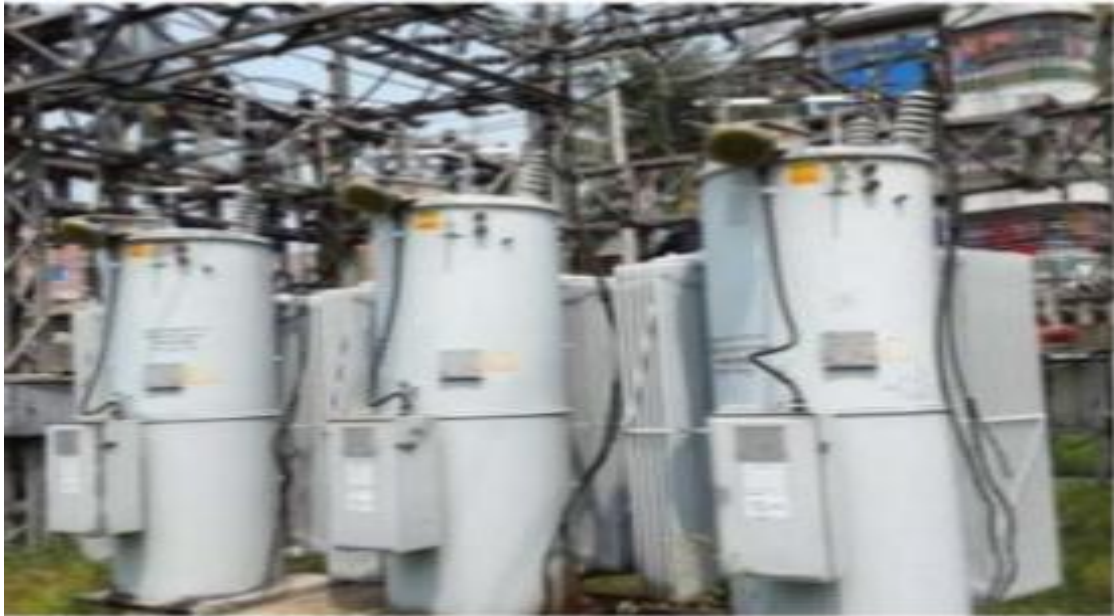
Figure: 3.5 Voltage Transformer
