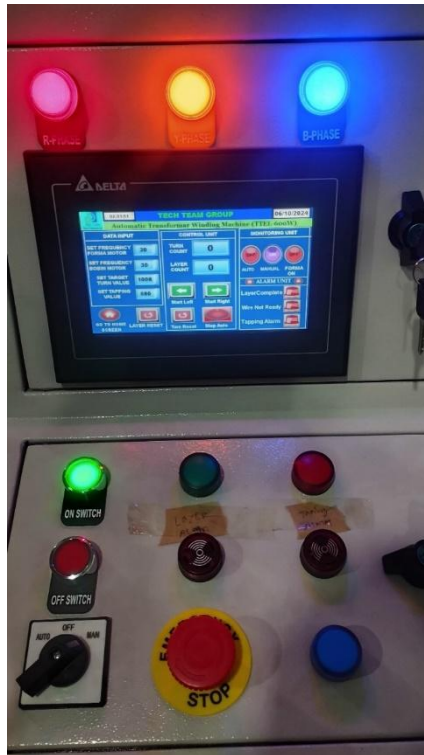
Figure 4.2. 1: Machine Parameter Setup in HMI and Operation Command Button.
