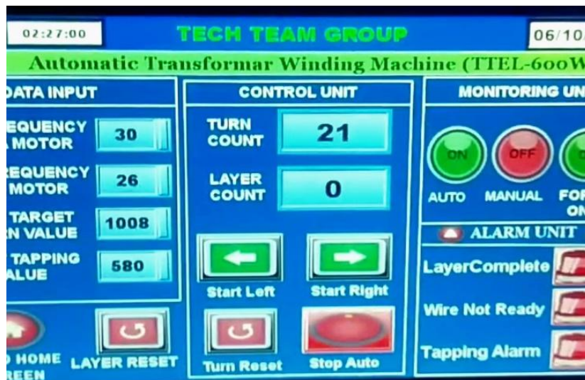
Figure 4.2. 3: Real Time Monitoring from HMI Screen.
