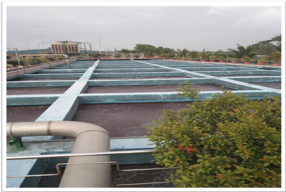
Figure 5: Biological Effluent Treatment Plant
