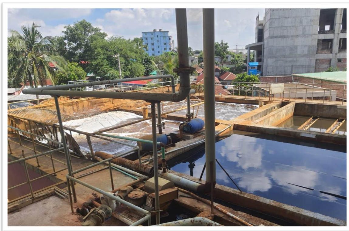
Figure 4: Bio-chemical Effluent Treatment Plant
