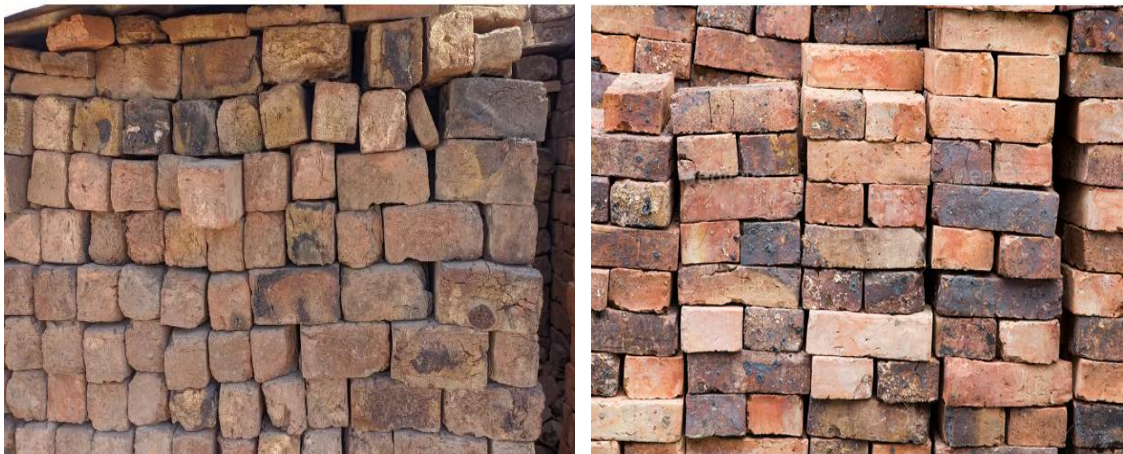
Figure 2.6: Over burnt Bricks
