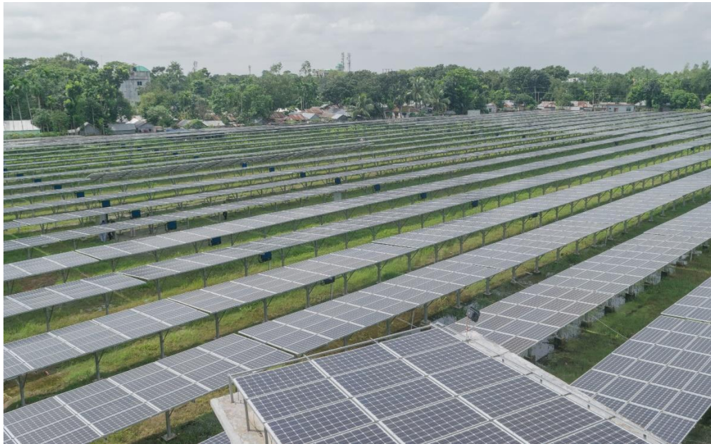
Fig2.7: Sarishabari solar power plant.
