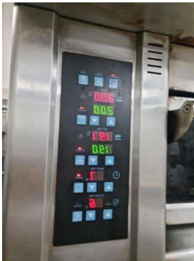
Figure 7: Control Panel of Deck Oven
