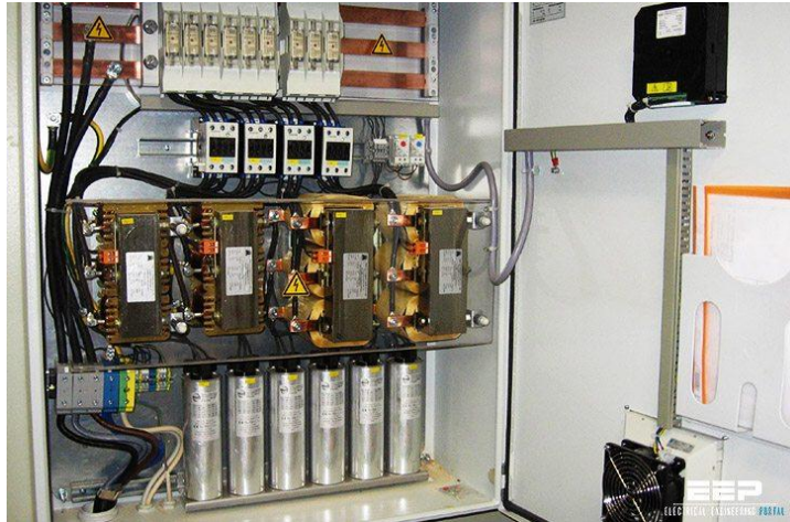
Fig 3.6: Automatic Capacitor Bank
