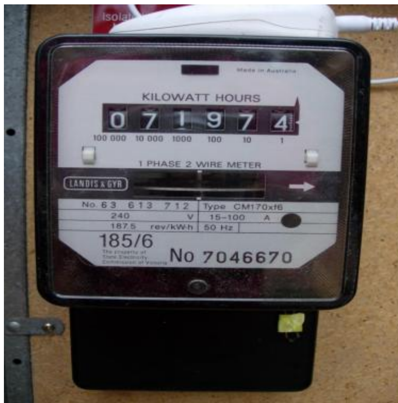
Figure 3.4: Traditional Electricity meter
