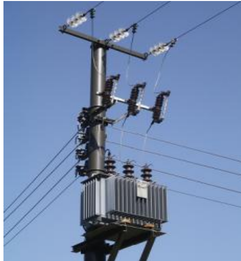
Fig1.4.2.e: Pole Mounted Substation
