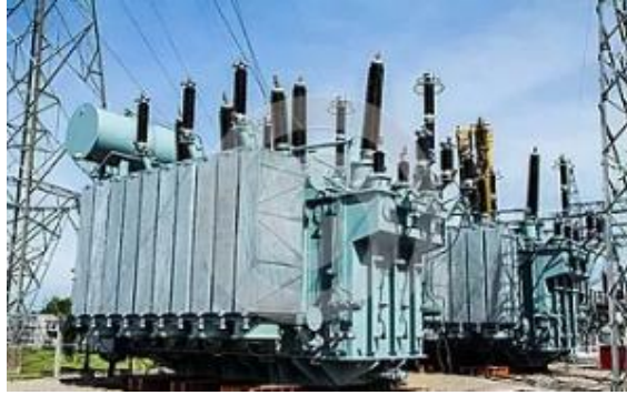
Fig1.4.1.b: Step Down Substation
