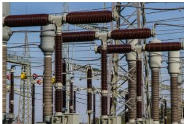
Fig1.4.2.b: High Voltage Substations
