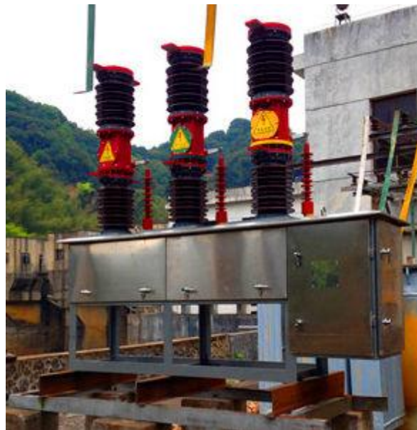
Fig:3.5.1.2.c: Outdoor Circuit Breaker
