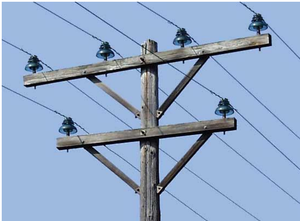
Figure 2.1: 11KV Transmission line
