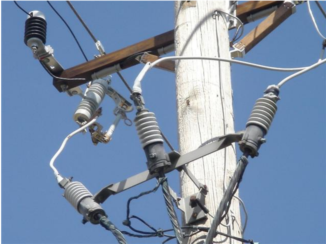
Figure 3.3: The 11KV Feeder III
