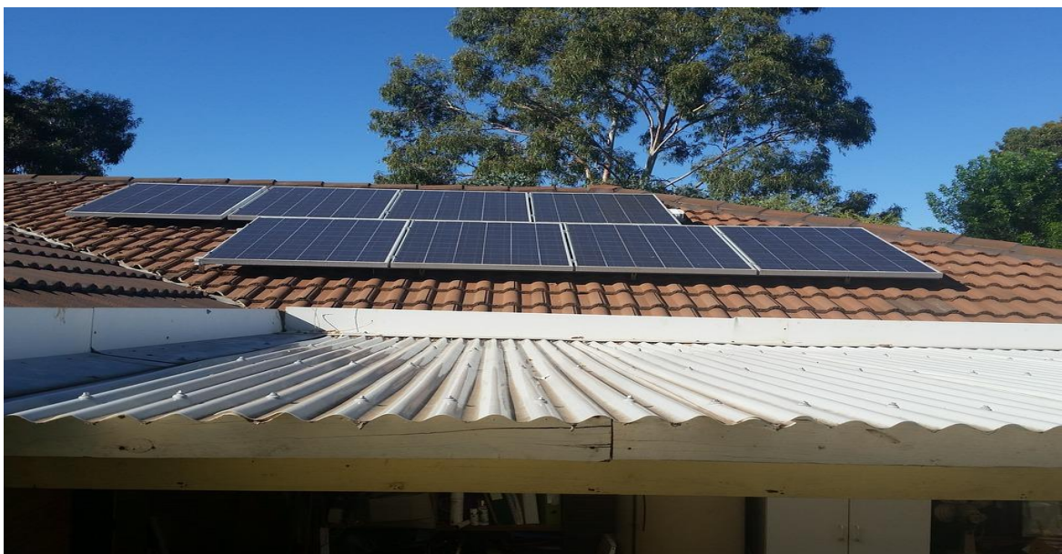
Fig-2.7: Rooftop Solar home system
