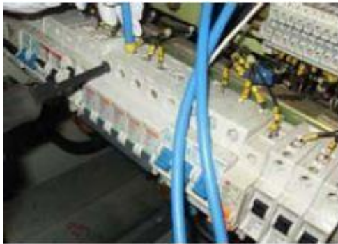
NEGATIVE POWER CABLE CONNECTION AT RECTIFIER END
