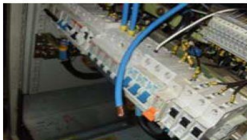
POWER CABLE CONNECTION AT RECTIFIER END
