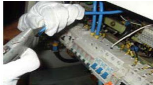
POWER CABLE CONNECTION AT RECTIFIER END
