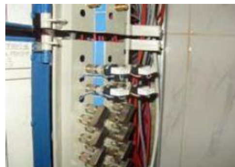
AFTER CROSS CHECKING E1 PATH CONNECT BALUN
