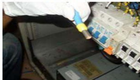
USE PROPER LUG FOR POWER CABLE
