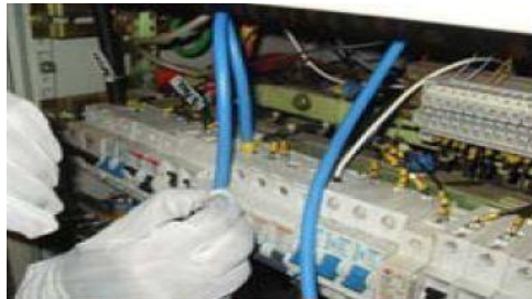
POWER CABLE CONNECTION AT RECTIFIER END
