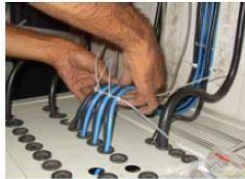
LATCHING THE POWER CABLE AT RECTIFIER END
