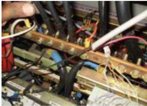
POSITIVE POWER CONNECTION for BTS & EMU AT RECTIFIER END
