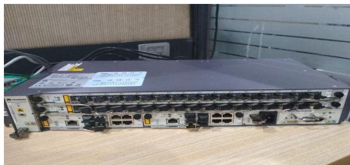
Fig 4.11: Optical Line Terminal (OLT)
