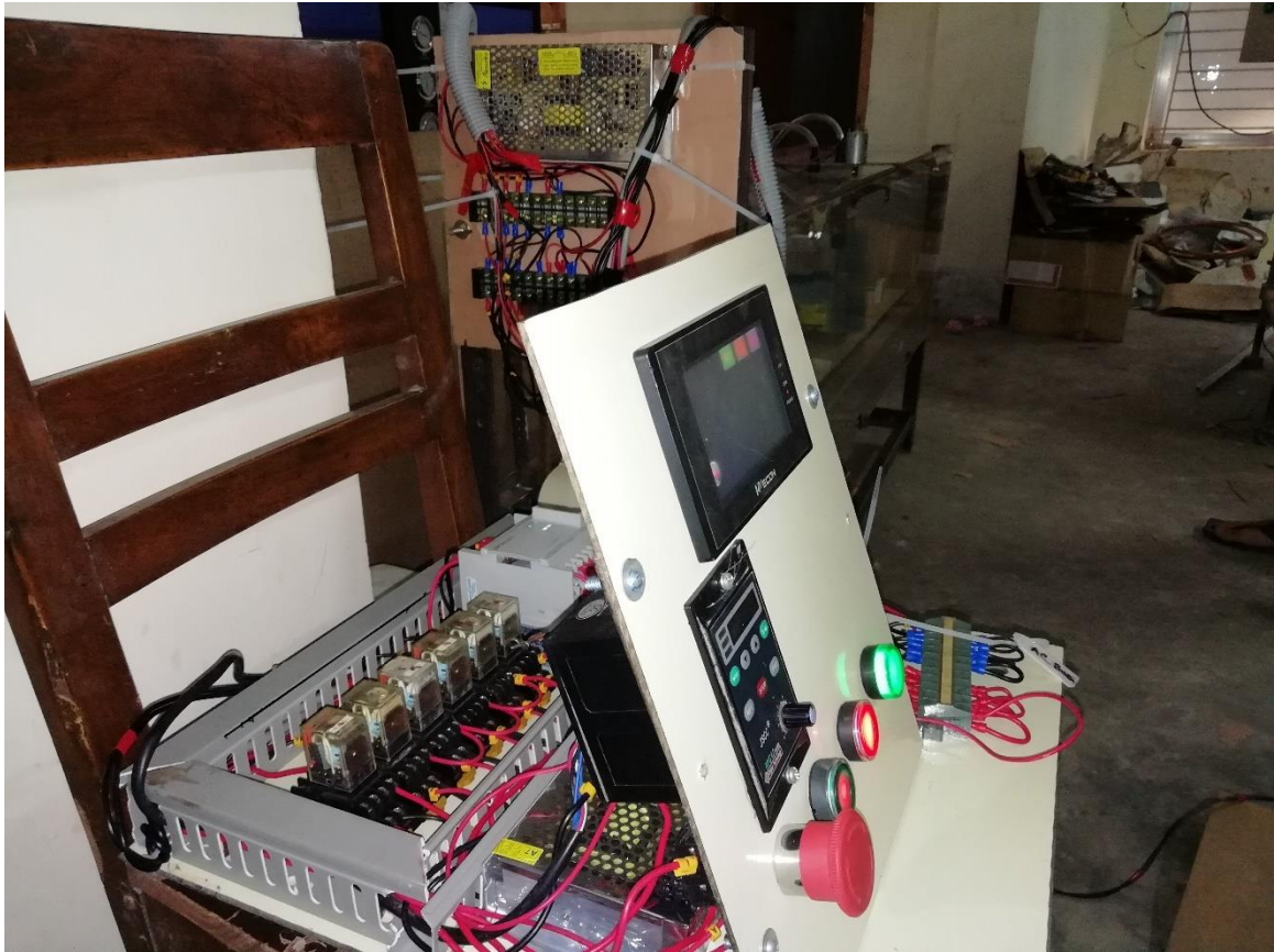
Figure 4-6 Main control panel
